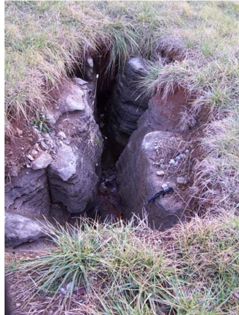
16 – Sinkhole between I-264 WB and I-64 EB Exit Ramp to I-264 WB
