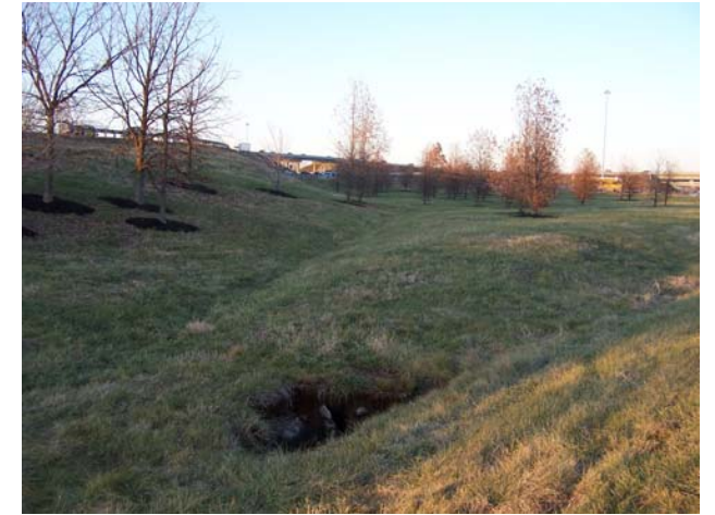
15 – Sinkhole Between I-264 WB and I-64 EB Exit Ramp To I-264 WB
